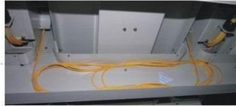
Fiber jumping passage
