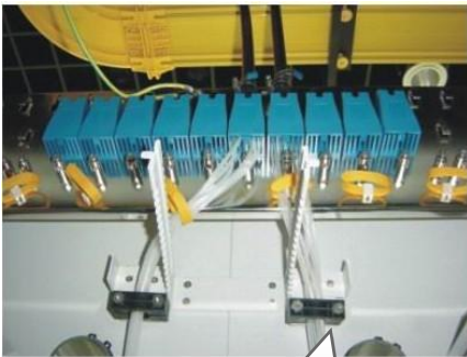
Optic cable inlet (single-layered structure)
