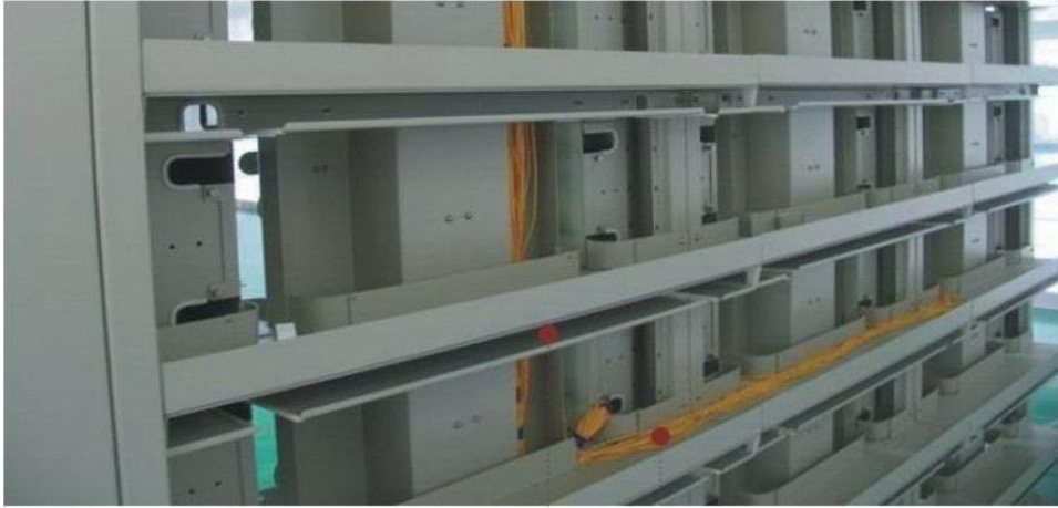
Rear fiber jumping and pigtail passage (double layer)
